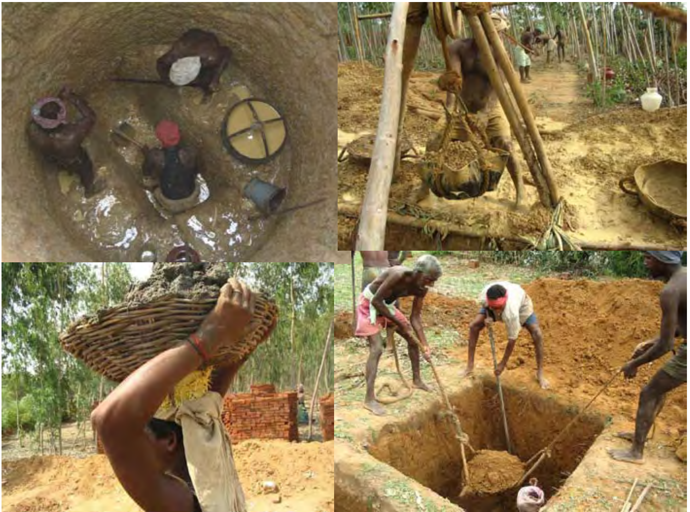
The construction of a new building for the Mother Teresa School in Periyakrishnapuram starts with digging for the water well and the foundations.
